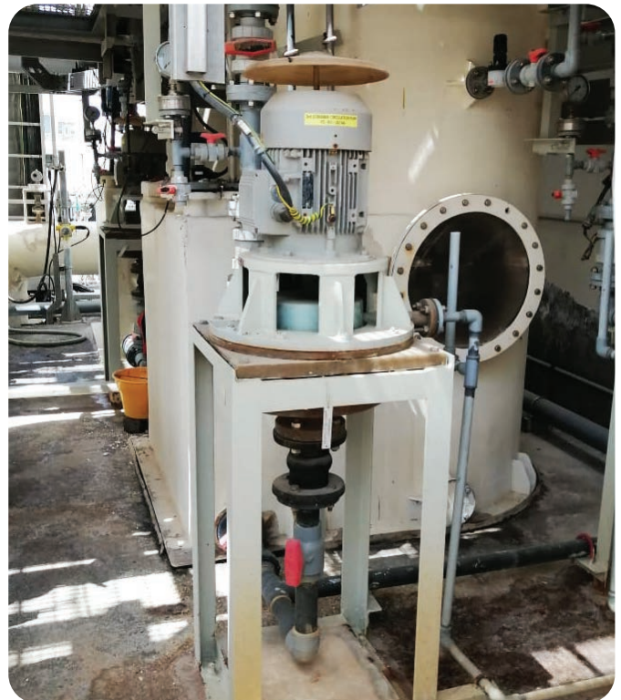
Existing circulation pump installation
