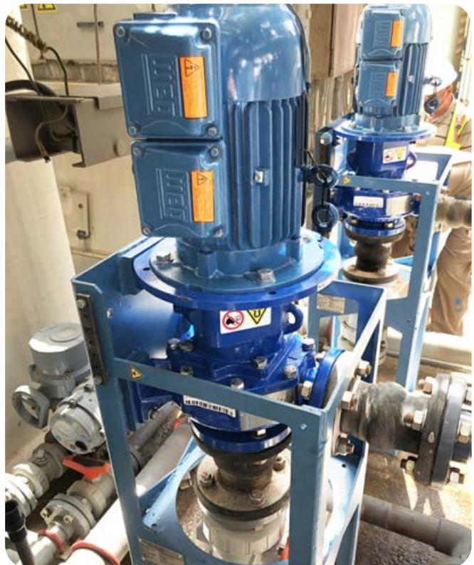
Installation of two INNOMAG TB-MAG sealless pumps with custom vertical mounting
