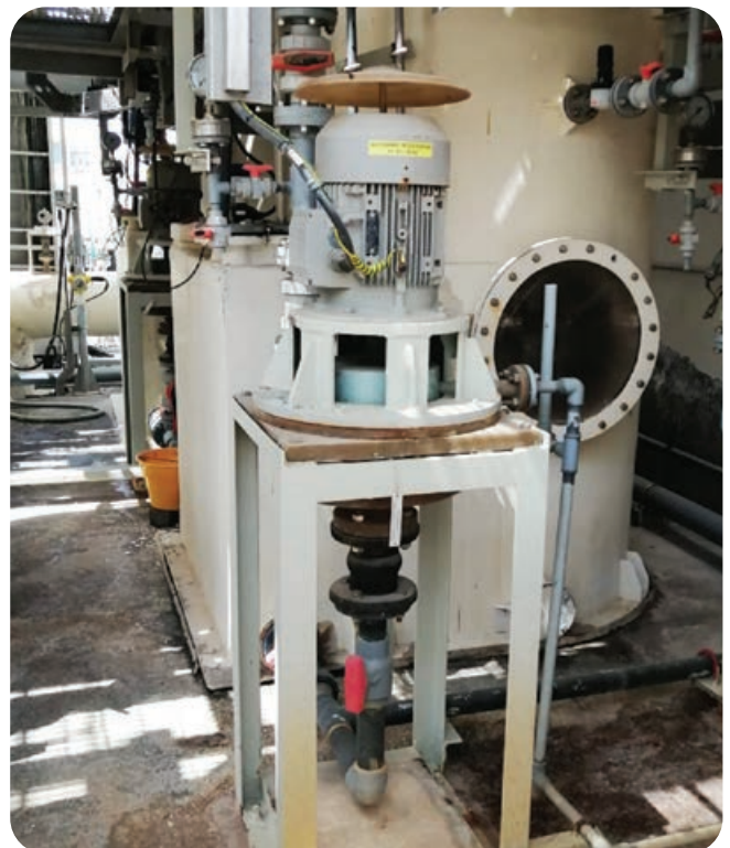
Existing circulation pump installation
