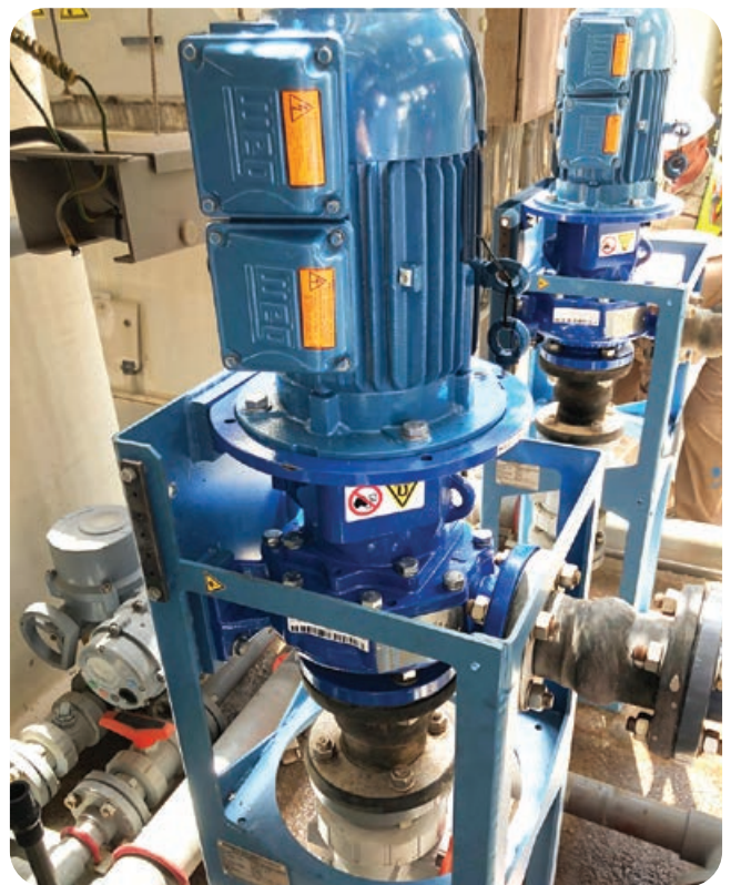
Installation of two INNOMAG TB-MAG sealless pumps with custom vertical mounting
