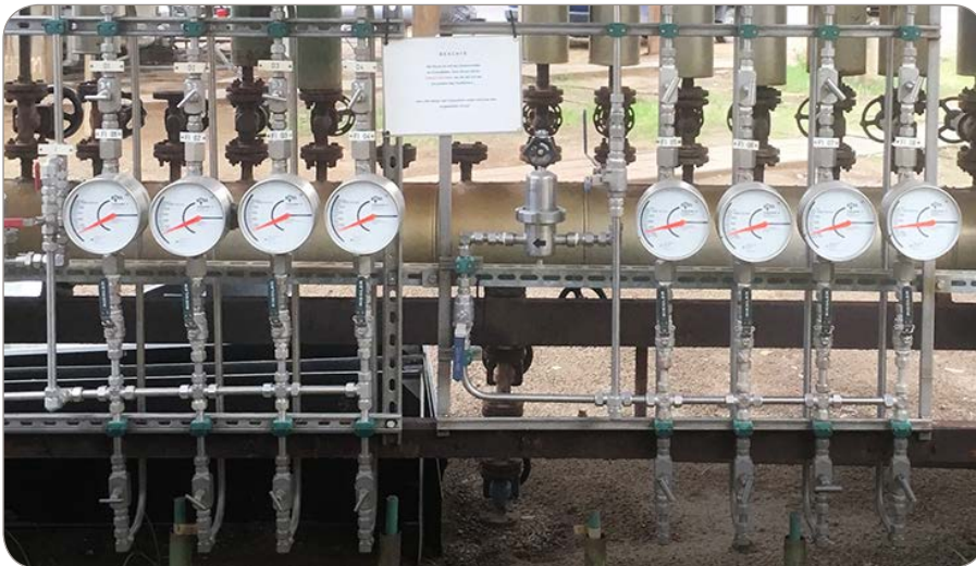
Front view of the barrier gas system controlling the Circpac LO seals of both blowers
