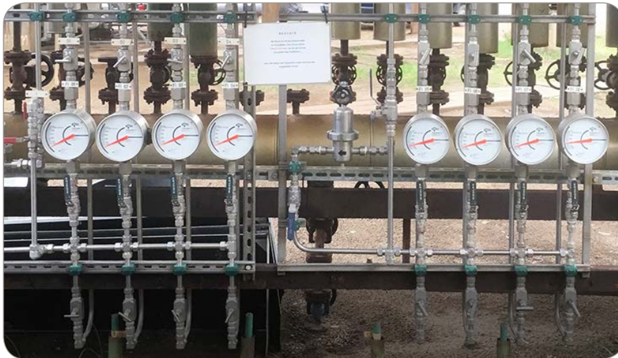
Front view of the barrier gas system controlling the Circpac LO seals of both blowers
