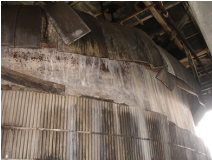
Leaking water from a competitor’s valve caused damage to the coke drum’s thermal insulation.
