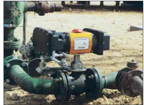
Oil production water dump application
