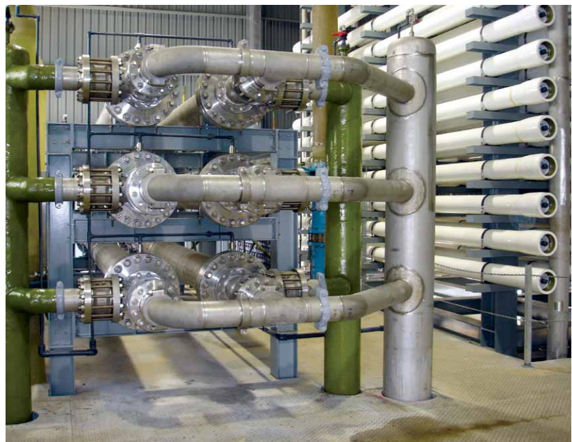
Figure 1. Dual work exchange energy recovery units for seawater reverse osmosis (SWRO) desalination can recover up to 98% of the energy in the brine waste system.
